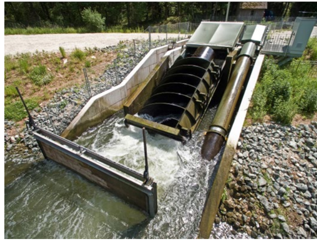
Hydropower by Screw Turbine
