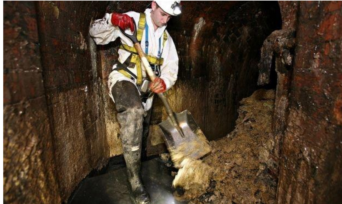
Fatberg causes severe damage in London sewer
