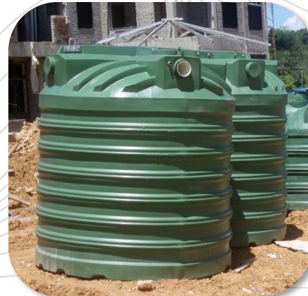
Individual septic tank
