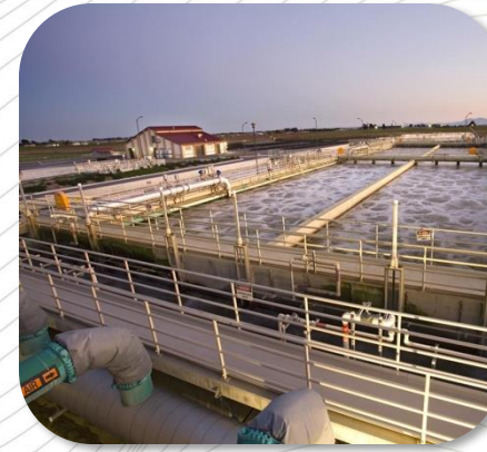
Water treatment system
